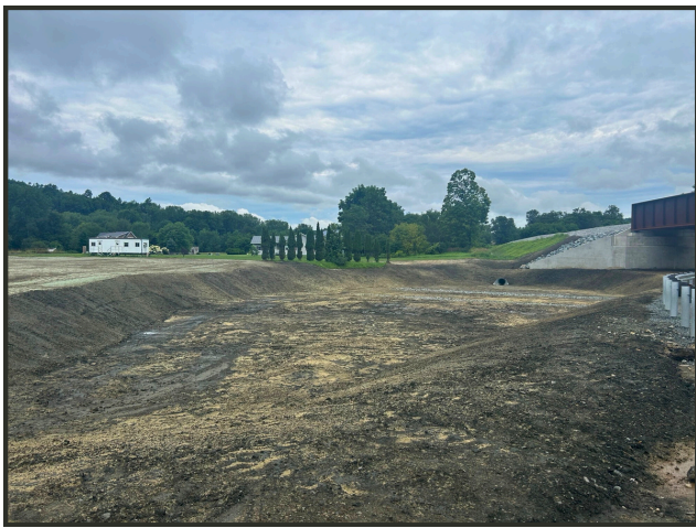
This retention pond alongside VT RT 14 has been re-lined with MFT in the beginning stages of the reclamation.
